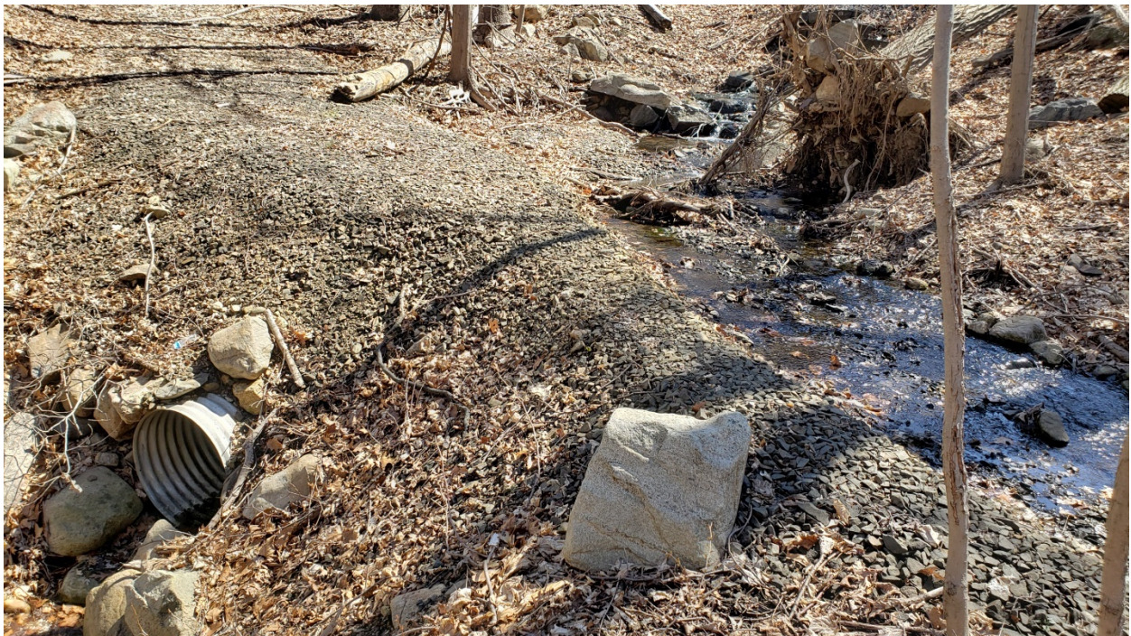
3/26/2019 Looking southeast at diverted Tributary 1 at compromised culvert
